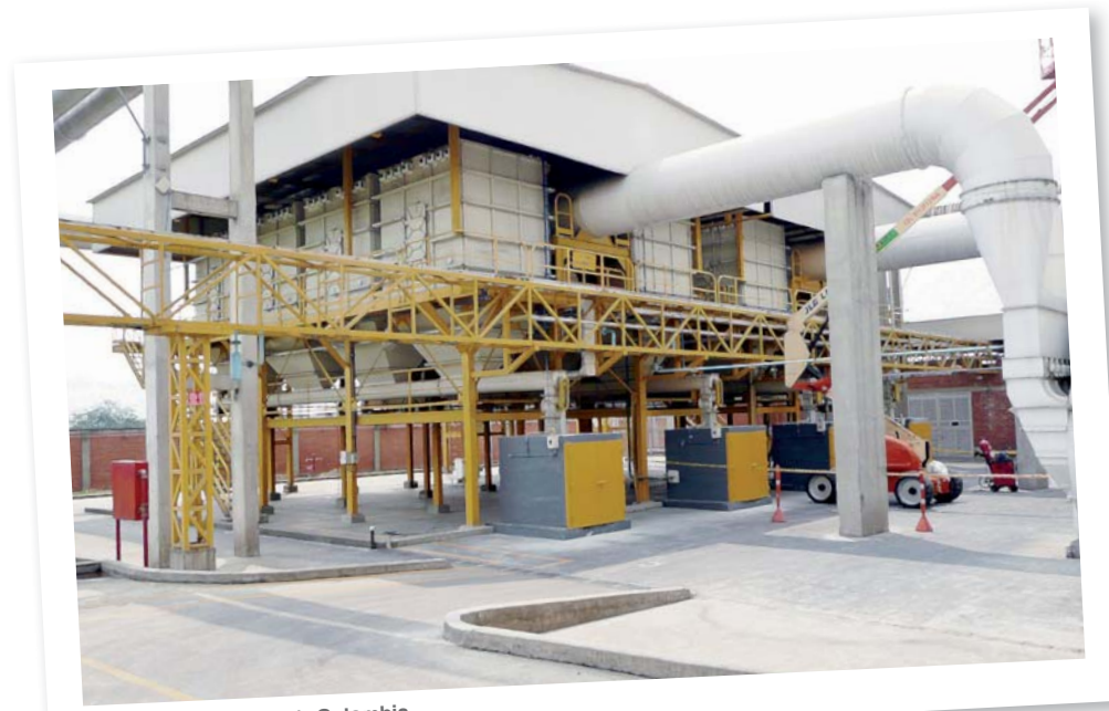
Filter Plant (Baghouse), Colombia
